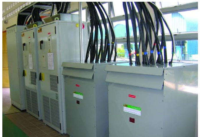
Layout of the pump controls (on left) and harmonic filters (on right).
