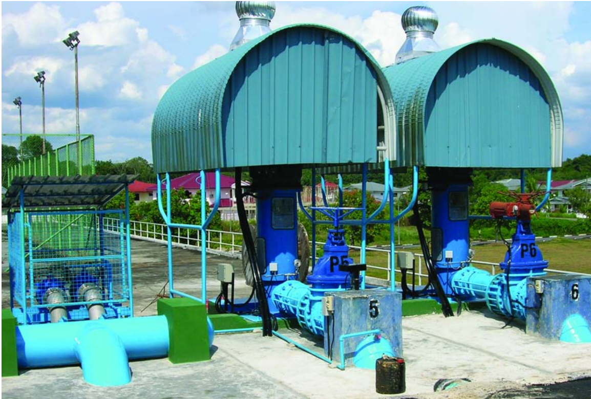
The Salim water treatment plant in Indonesia uses intelligent VFDs to control the lead-lag operation of these new replacement pumps. On the left is the surge valve that replaced the surge vessel to avoid water hammer.
