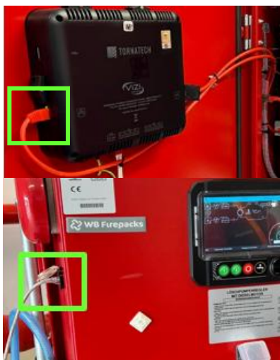
Main Fire Pump Controller
